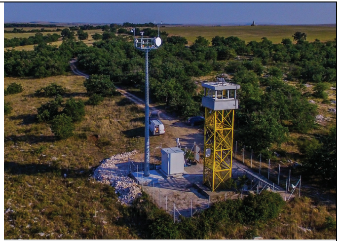
A total of six stations have been installed, complete with a FLIR Triton PT-Series HD, weather station, a solar power array, and a microwave transmission system.
